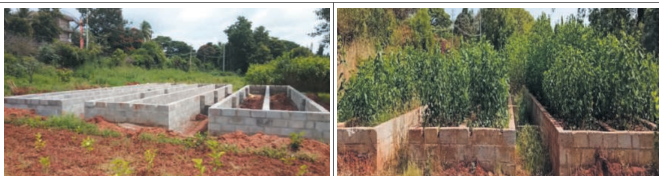
Constructed 3 nos. of root structures (cement structures) and established plantation of diverse germplasm accessions in these structures
