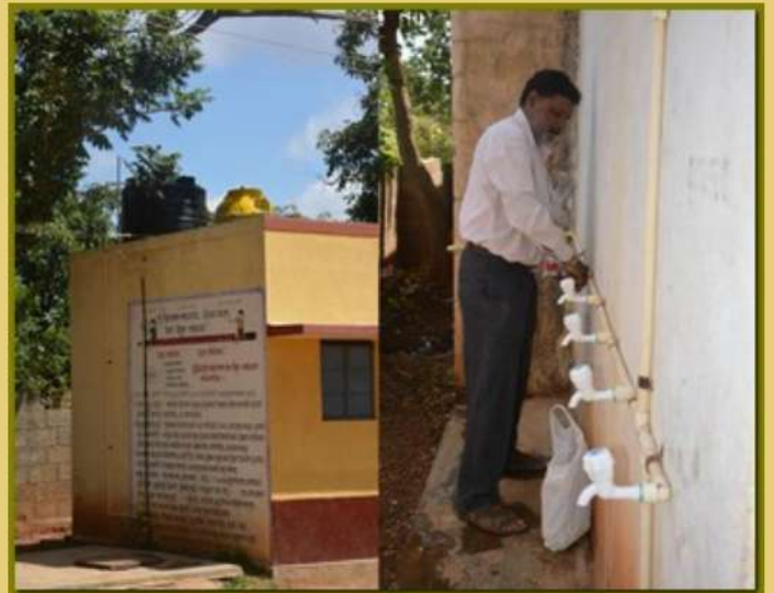
Commissioning of overhead tanks and taps for ensuring water supply to kitchen and toilets of the school
